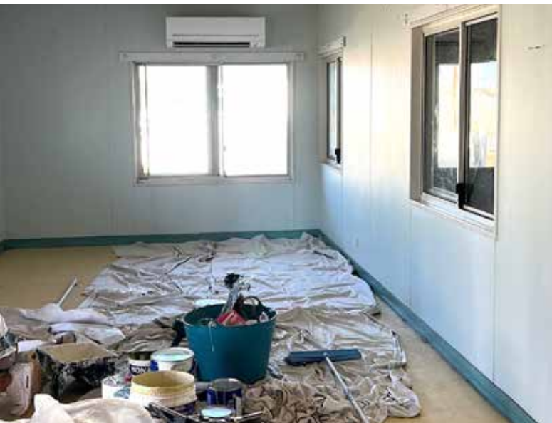
Freshly painted interiors, doors and replacement locks were part of the maintenance works completed by Bugardi Contracting in June 2023
